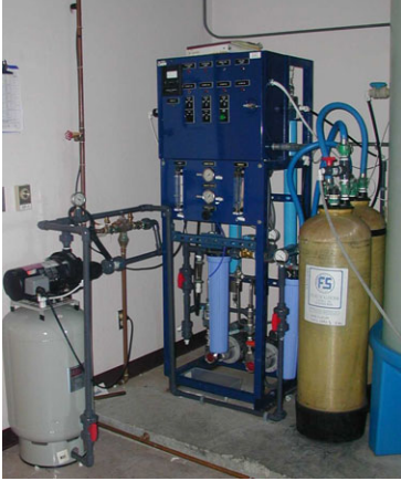
RO/DI Water Filtration System
