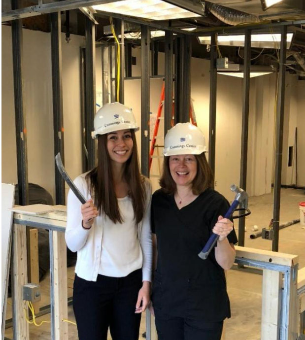
Dr. Audra Reynoso (left) with Dr. Lisa Campanella (right) of North Shore Pediatric Dental during the buildout of the orthodontic office.
